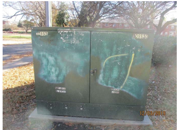
Photograph 16. View of the pad-mounted electrical transformer on-site.
