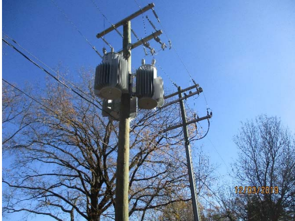
Photograph 17. View of pole-mounted electrical transformers on-site.
