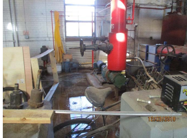
Photograph 10. View of the pooled water within the maintenance facility (observed dripping from overhead pipe – appears to be condensate).
