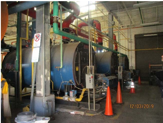
Photograph 7. View of the boiler heating system within the maintenance facility.
