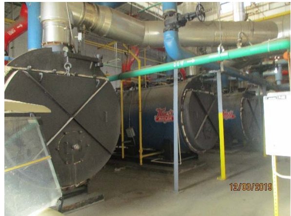
Photograph 8. View of the boiler heating system within the maintenance facility.
